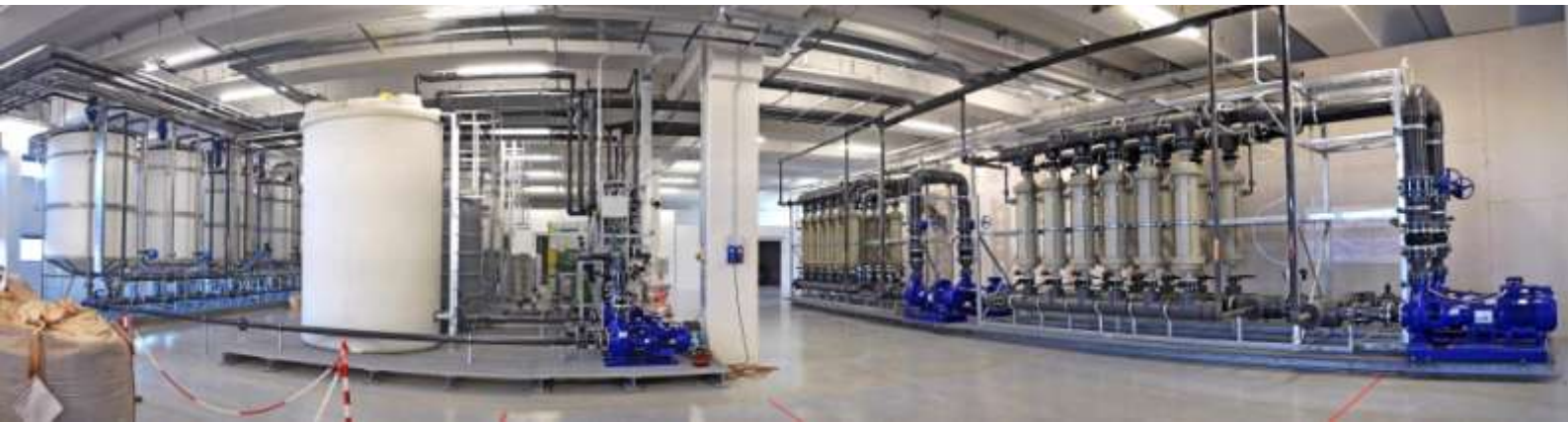
General View of the Plant
